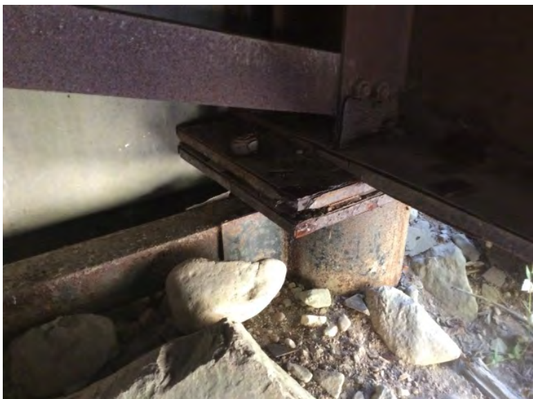
Bearing - townside corroding bearing
