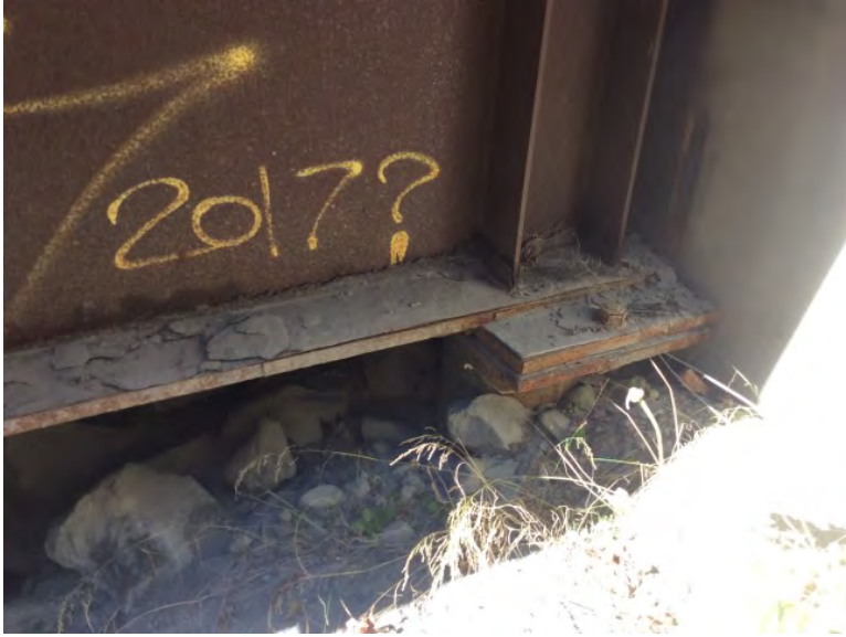
Bearing - u/s woodside corroding bearing plates
